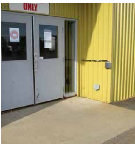
KA 6 | Power Door Control at Entrance
