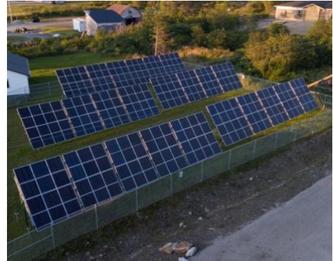
Figure 9: Administration Building Solar Field
